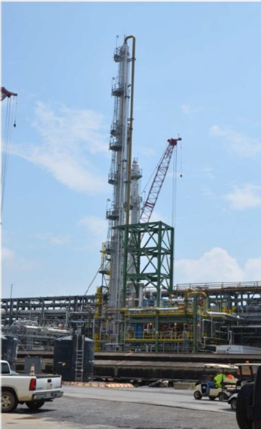
OASE® blue Pilot Plant at Wilsonville, US Capacity: 30 TPD CO 2 capture
