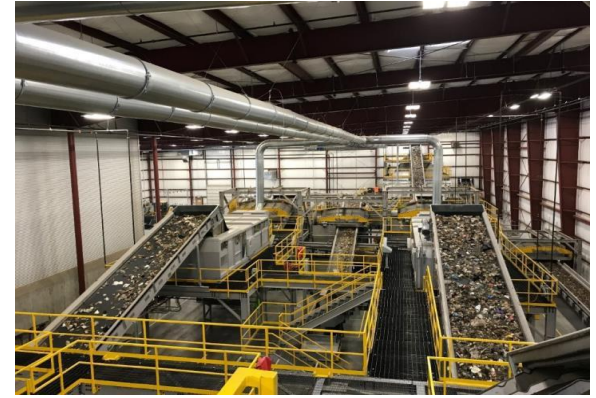
Fulcrum Sierra feedstock processing facility [courtesy Fulcrum Bioenergy]
